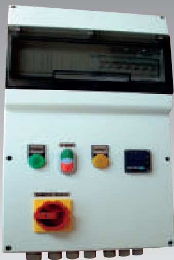
Control and power supply unit
