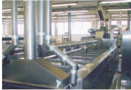
Industrial vessels and storage tanks
